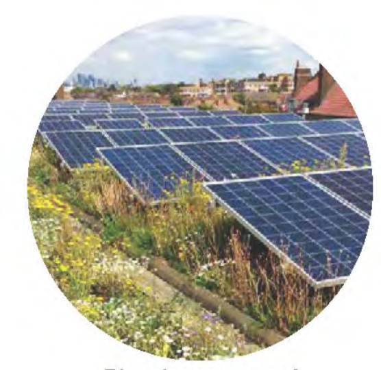
Biosolar green roof
